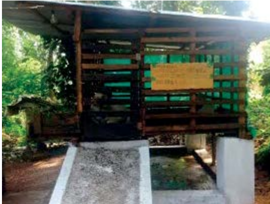
Goat shed constructed by MGNREGS women workers in Pallom Block, Kottayam District
